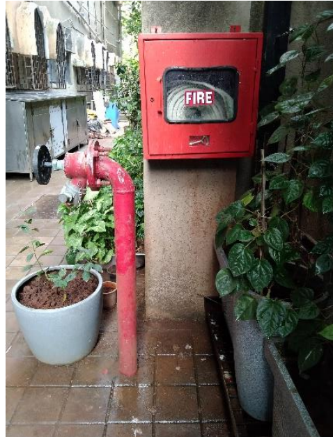
Fire Safety Equipments
