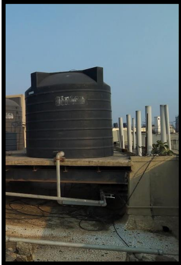
Water Management System on campus
