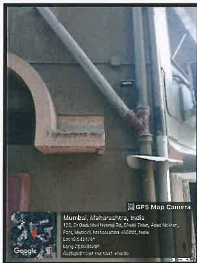
Network of water pipes
