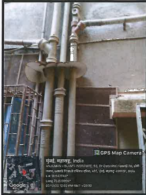
Drainage Pipes transporting waste water
