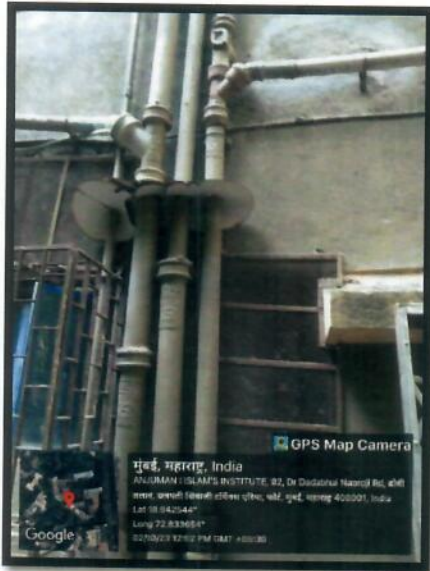
Pipes Carrying Water
