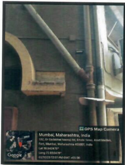
Network of water pipes
