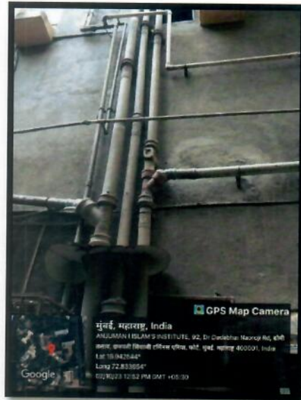
Pipes Carrying Water
