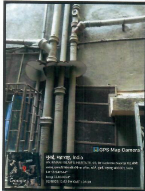
Drainage Pipes transporting waste water
