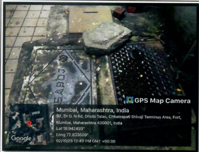
Drainage & sewer ducts
