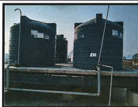
Water Conservation Tanks
