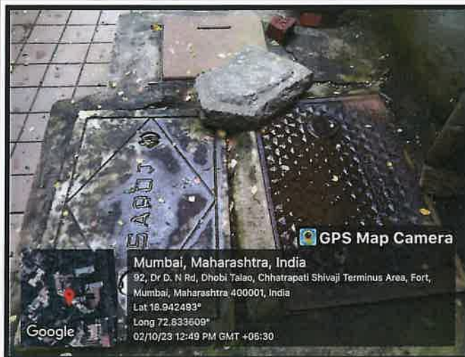
Drainage & sewer ducts
