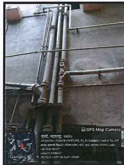
Pipes Carrying Water
