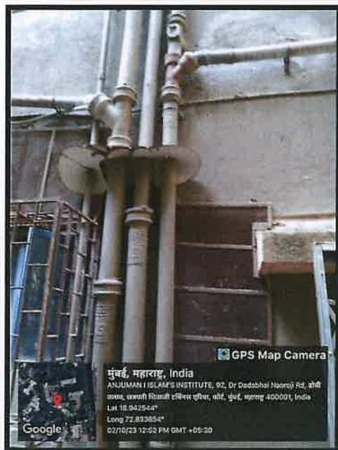
Drainage Pipes transporting waste water
