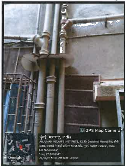
Pipes Carrying Water
