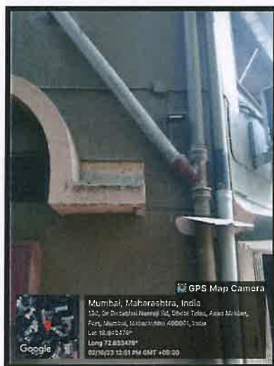
Network of water pipes
